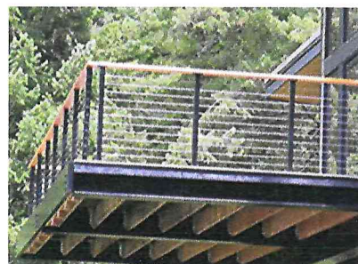
Fig. 5 Example of stainless railing sys.
